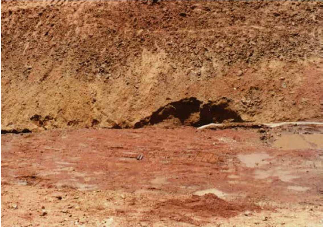
Picture 5 Upstream parallel cut-off bottom showing mainly pink pegmatite below sand layer at RD 1463m (Ch 48) on left bank.
