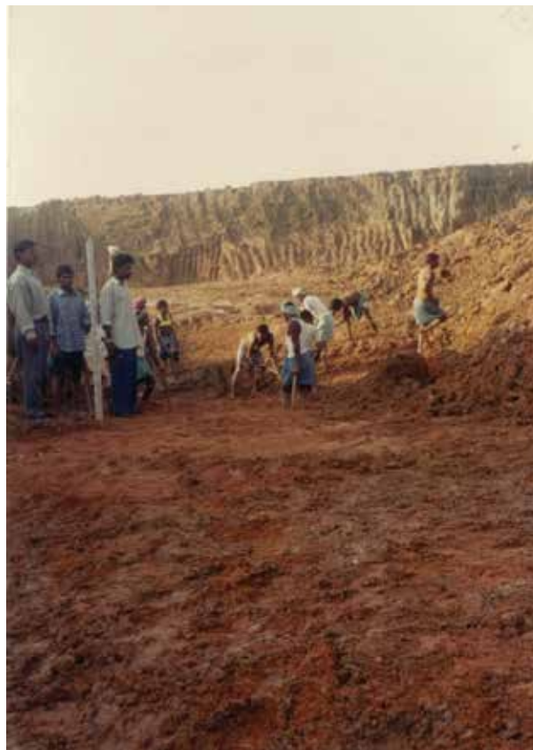
Picture 4 Upstream parallel cut-off bottom showing granite gneiss intruded by pink pegmatite below sand layer at RD 1509m (Ch 49.5) on left bank.
